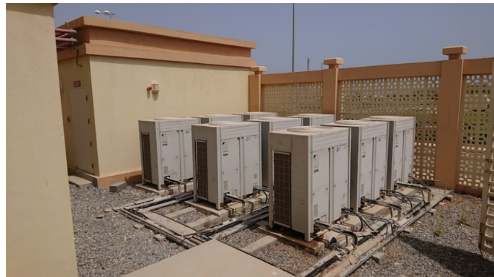
Image 2. Split air conditioning units are monitored and can be controlled on occupancy, temperature or other environmental data to reduce energy use and improve comfort levels
