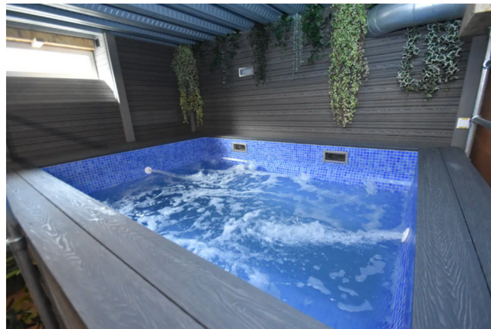
Image 2. The hot tub is fed by one of the twin boilers
